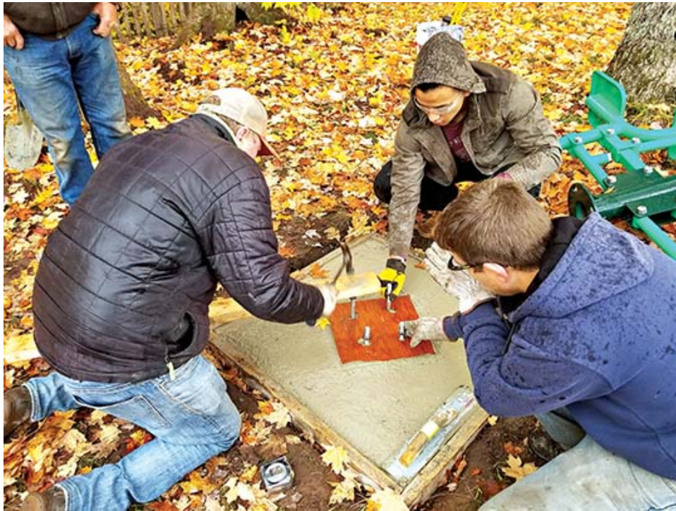
(Photo provided by the Chassell Township) Planning Commission Dan Palosaari, Will Hagelthorn and Pete Torola setting J-bolts into a concrete foundation with a template developed by Dennis Karvakko.
